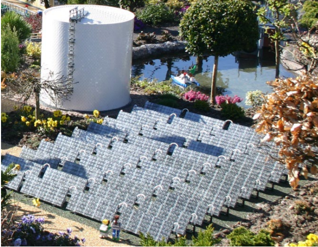
Tank heat storage (TTES)
